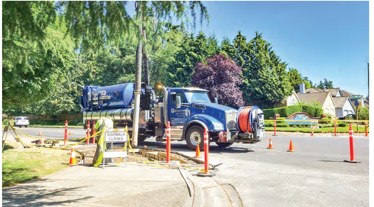
Mukilteo Public Works crew installing sidewalks on Harbour Pointe Blvd on August 2, 2022. Lynnwood Times | Mario Lotmore.
